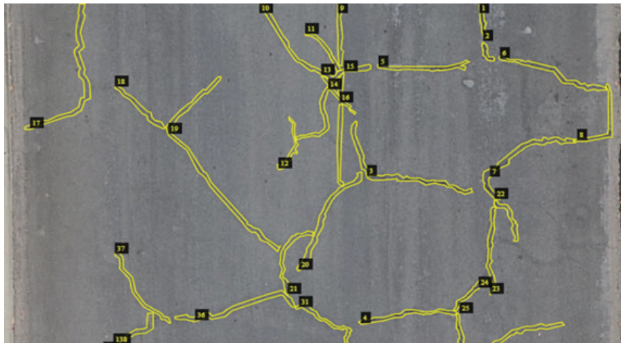
Figure 1. Sample Annotation of Roadway Damage using VGG Image Annotator (VIA).
